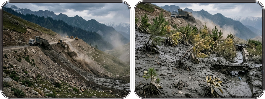
Muck dumping and damage to vegetation and plantation along the slope
